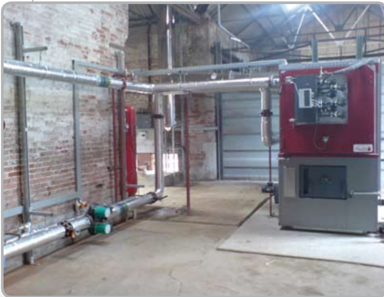
Above: The Gilles HPK-UTSK 550kW in the central boiler room converted from an old grain store is at the centre of the system.
